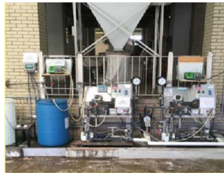
Photo 2: Temporary pump/metering system for the application of corrosion chemicals.
