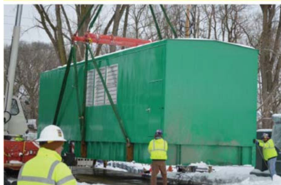
Photo 2: Typical generator housing installation at a water/wastewater treatment facility.
