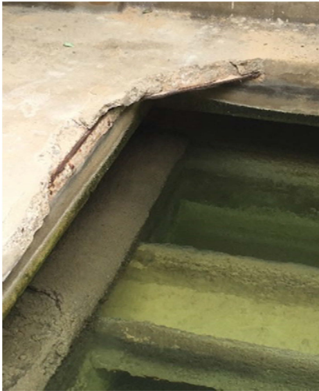
Photo 1: Photograph of the condition of the existing concrete walkways and support beams associated with the plant sand filter.
