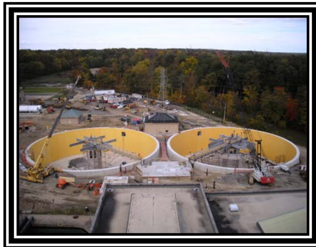
Photo No. 1 – Solid Contact Clarifiers
